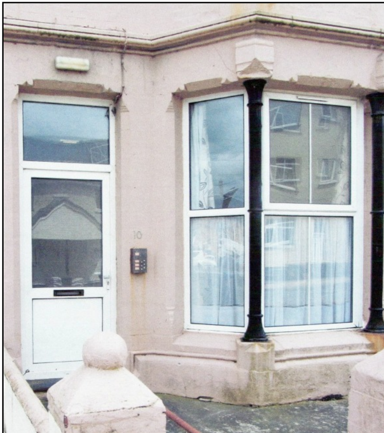
LEFT The carving of the sandstone dressings around the window has survived better than on other houses in the Terrace, and shows the craftsmanship used for these houses. The columns are iron.
