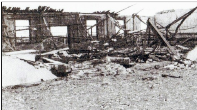
ABOVE A photograph from Y Tincer, June 1993 shows extensive damage to the building.
