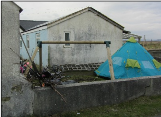
LEFT The south gable end of the bungalow has a small window which looks over an enclosed yard, with a wall between it and the lane which turns past it there.
